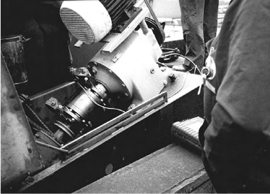
Water Treatment Installation
